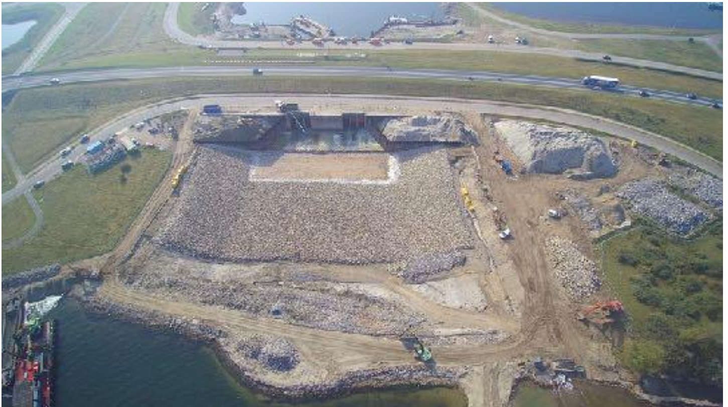
Tidal Technology Center Grevelingendam (foto: BT Projects)
